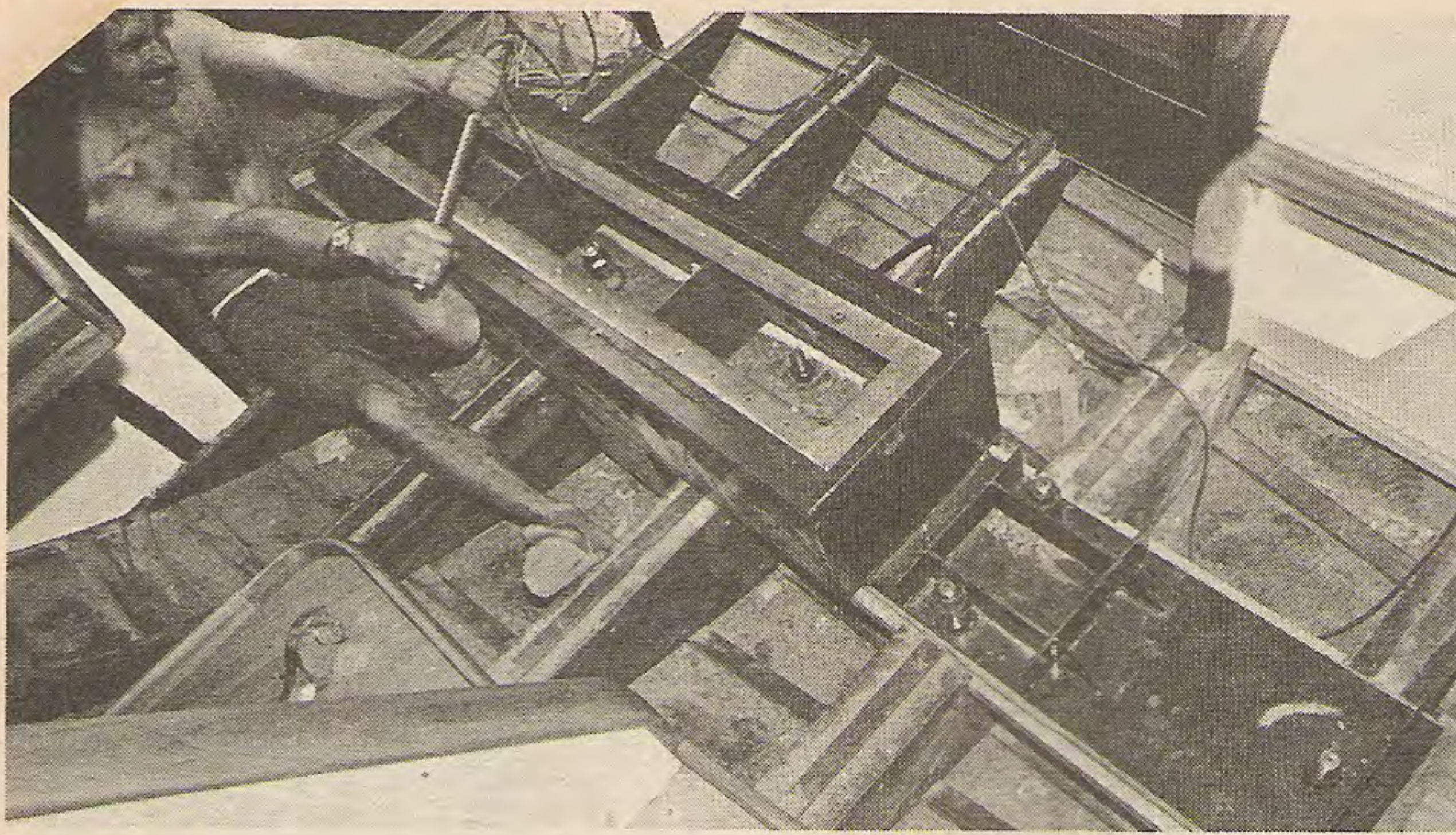
Don Senior tightening the keel bolt nuts in the fabricated steel unit that, with its top on, acts as the fuel tank, the extension forward also being the mast step. The whole is covered by a central "island" sink bench and ice-box unit
